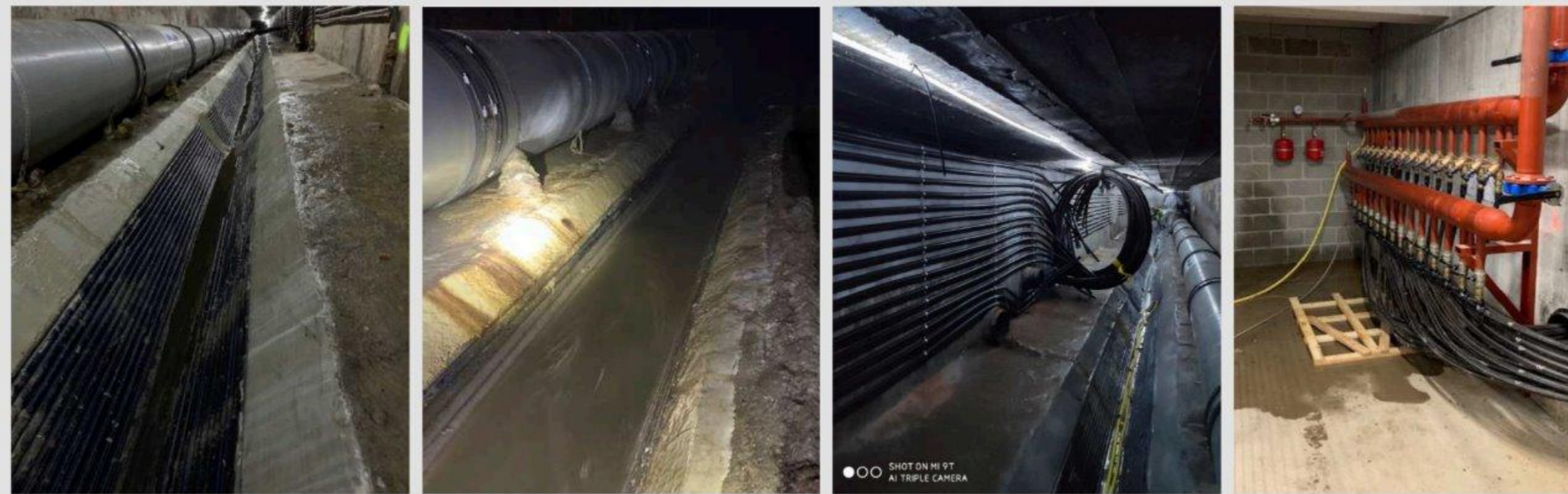
In-sewer heat exchangers
