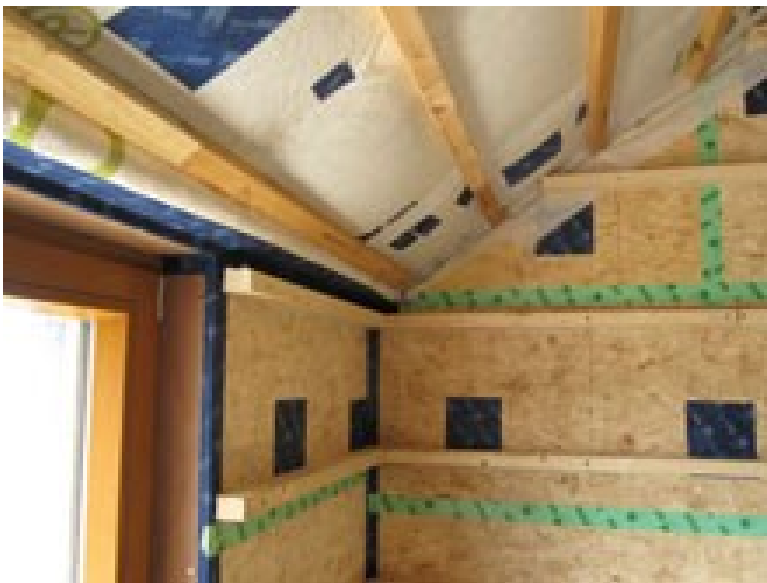
Raccords divers Source: Buildwise
